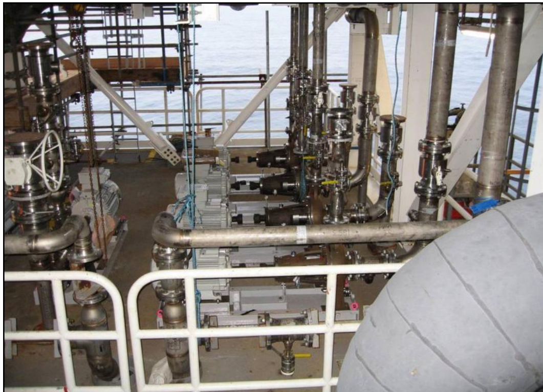
Pumps in situ between decks
